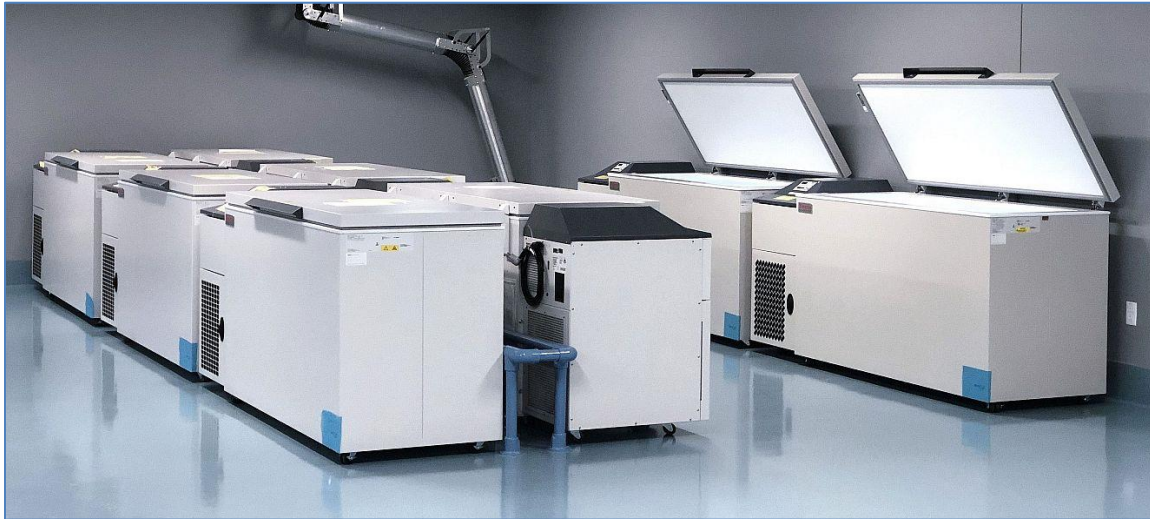
Inside the new freezer farm at Vetter's US Development Service site. Picture source: Vetter Pharma International GmbH
